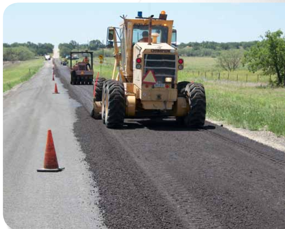
TxDOT Abilene District crew overlaid several miles of FM 2287 near Cross Plains with PASS-R, a new design of solvent-free recycled asphalt pavement (RAP) developed by Western Emulsions, Inc.
